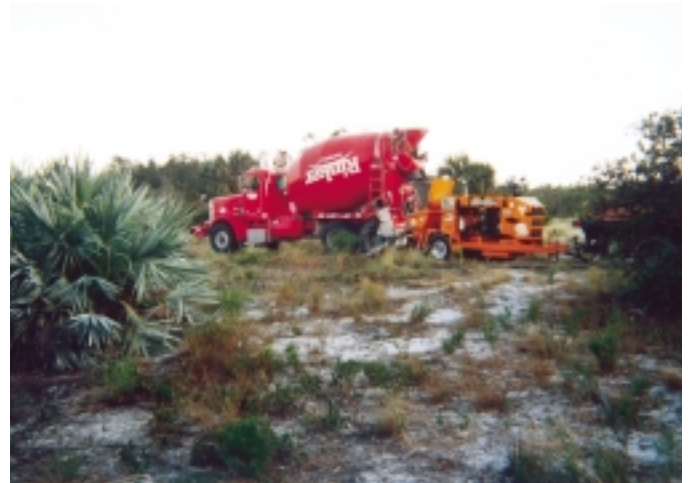
A Putzmeister Katt-Kreter™ trailer-mounted concrete pump undertook the major challenge of pumping concrete through two-inch rubber hose at extremely long distances of 1000-ft.
