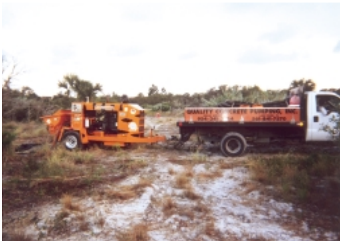
Quality Concrete Pumping of Coral Springs, FL was relied upon to expertly handle the concrete mix so it didn't get stuck in the long 1000-ft hose needed when pumping three pours that totaled 200 cubic yards.
