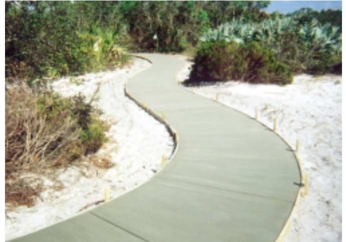
One aspect of the project involved construction of a winding 1,900 linear feet long concrete sidewalk, designed to keep visitors off the scrub.
