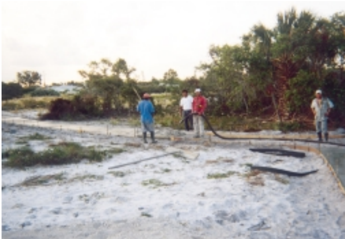
It was imperative to keep concrete and hose within the forms to avoid disruption to the sensitive habitat.
